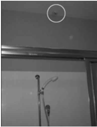
Figure 2: Motion sensor installed above the shower to detect bathing activity.
